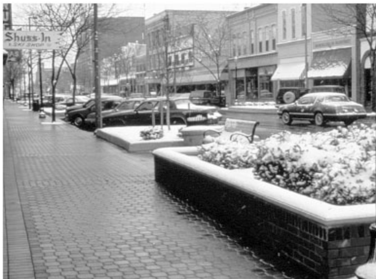
Figure 1. A snow melting system under concrete pavers in downtown Holland, Michigan has performed well since 1988.
