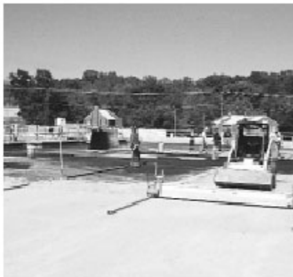
Figure 18. A mechanical screed used to level bedding sand on a roof parking deck project.
