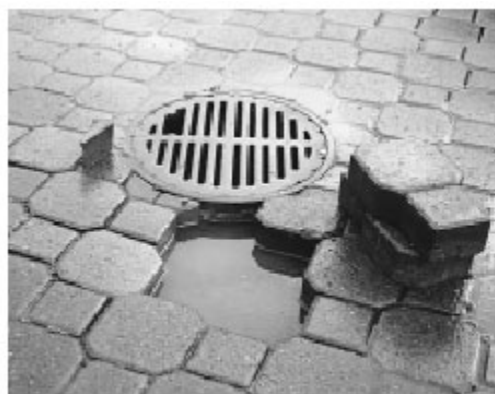
Figure 15. An absence of holes in the sides of this roof drain led to ponding.
