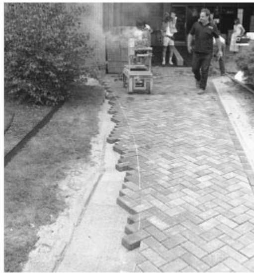
Figure 15. Saw cutting marked pavers on bedding sand. The cut pavers are carefully removed and edging is placed against the pavers and spiked in place.
